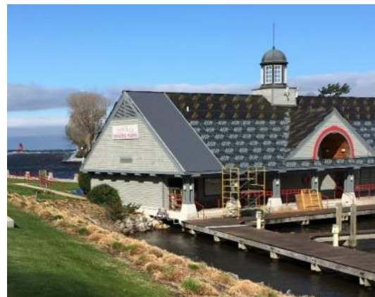
Figure 27: New steel roof installation example; City of South Haven, South Side Marina
