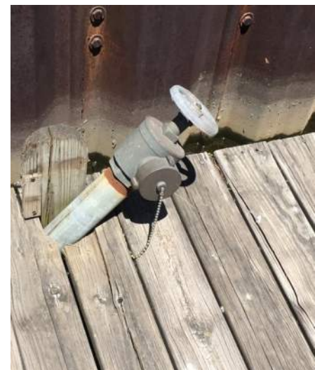
Figure 15: Dry standpipe hydrant
