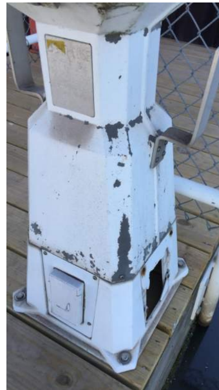
Figure 12: Damaged utility pedestal
