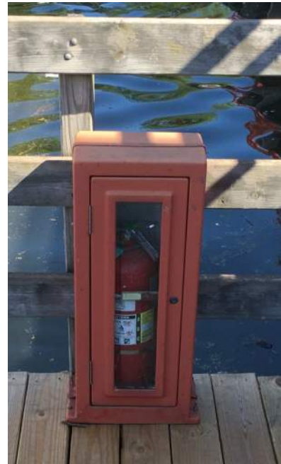
Figure 14: Typical Fire Extinguisher cabinet
