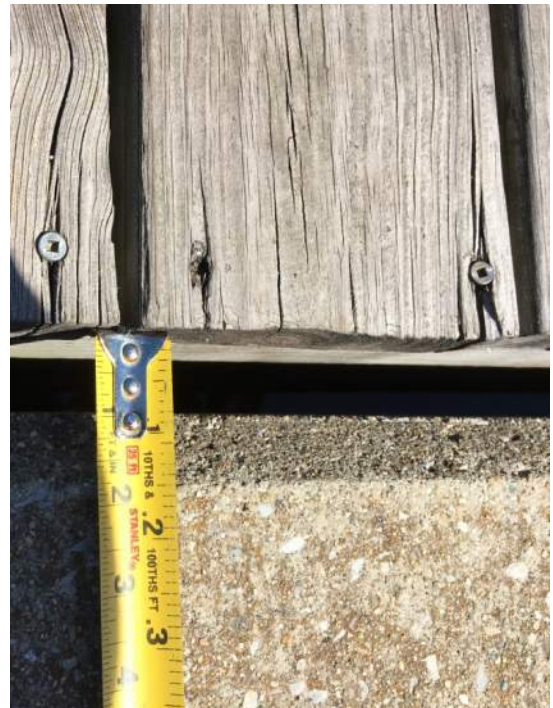
Figure 6: Gangway platform gap
