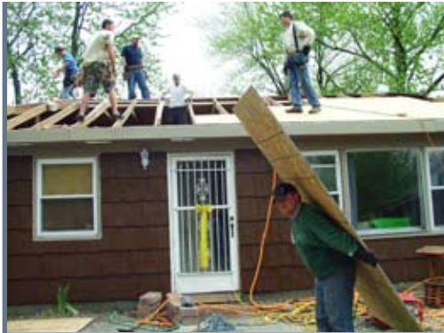
The nonprofit organization, Rebuilding Together, install a new roof on a home in Portage. The organization's mission is to preserve affordable homeownership and revitalize communities.
